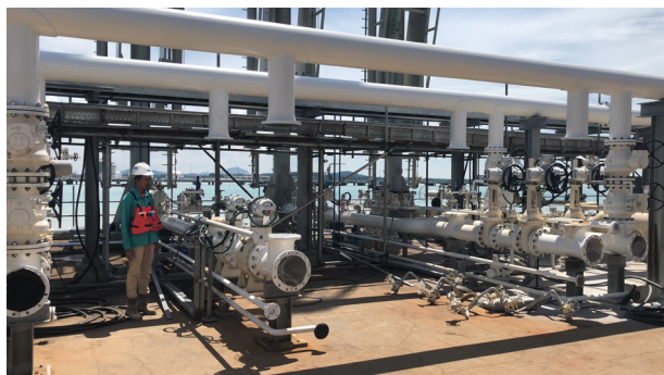
Figure 1. Intelligent actuators in operation at a terminal.
