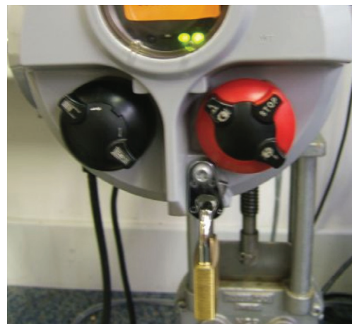
Fig 3 IQ/IQT control selector padlocked in "Remote"
