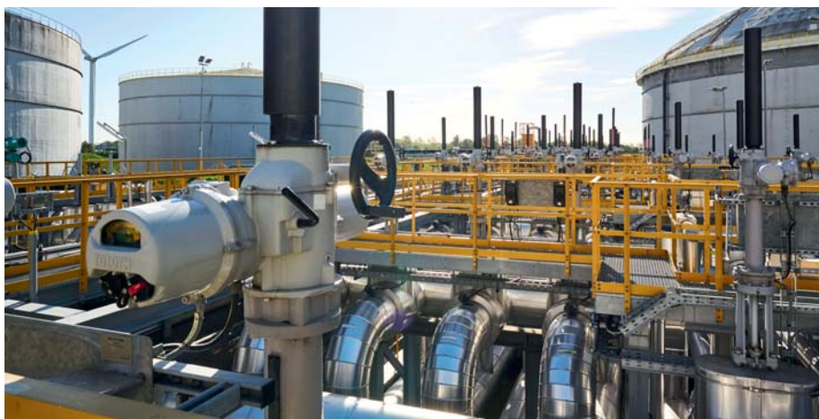
Intelligent actuators on site at a terminal
