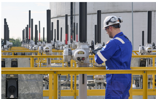
Figure 3. A Rotork service engineer carrying out a health check.
