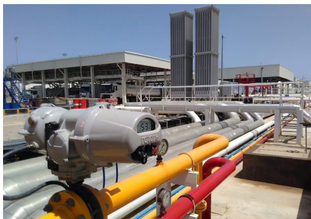
Figure 1. An actuator onsite at a fuelling depot.
